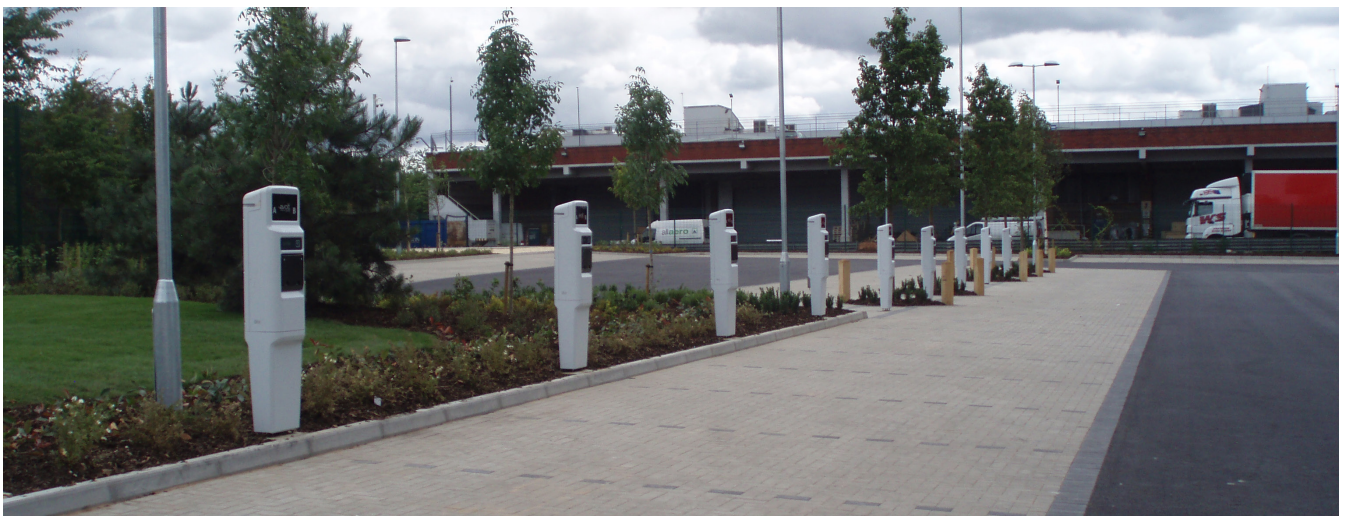
Example of several Circontrol's Charging Solutions installed at Heathrow (UK)
